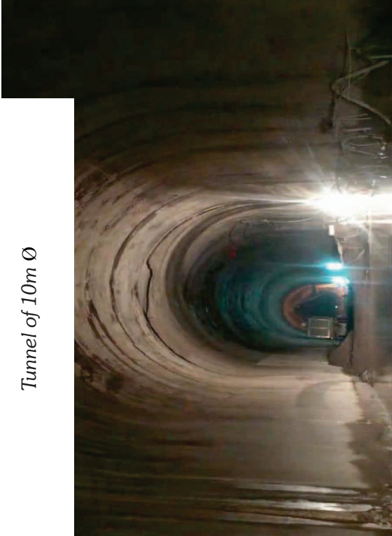
Gayatri Pump House
