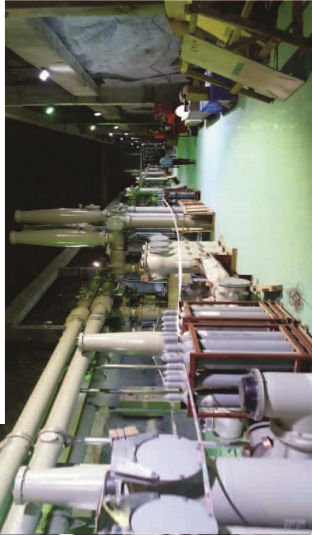
400 KV underground Gas Insulated Sub Station at Nandi Pump House
